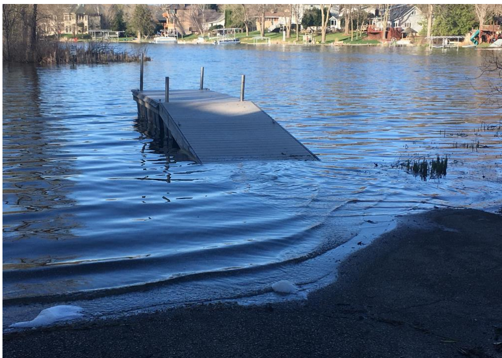
Flooded boat-launch southeast bay – April 24, 2019 Note concrete walkway under water leading to floating launch pier.
